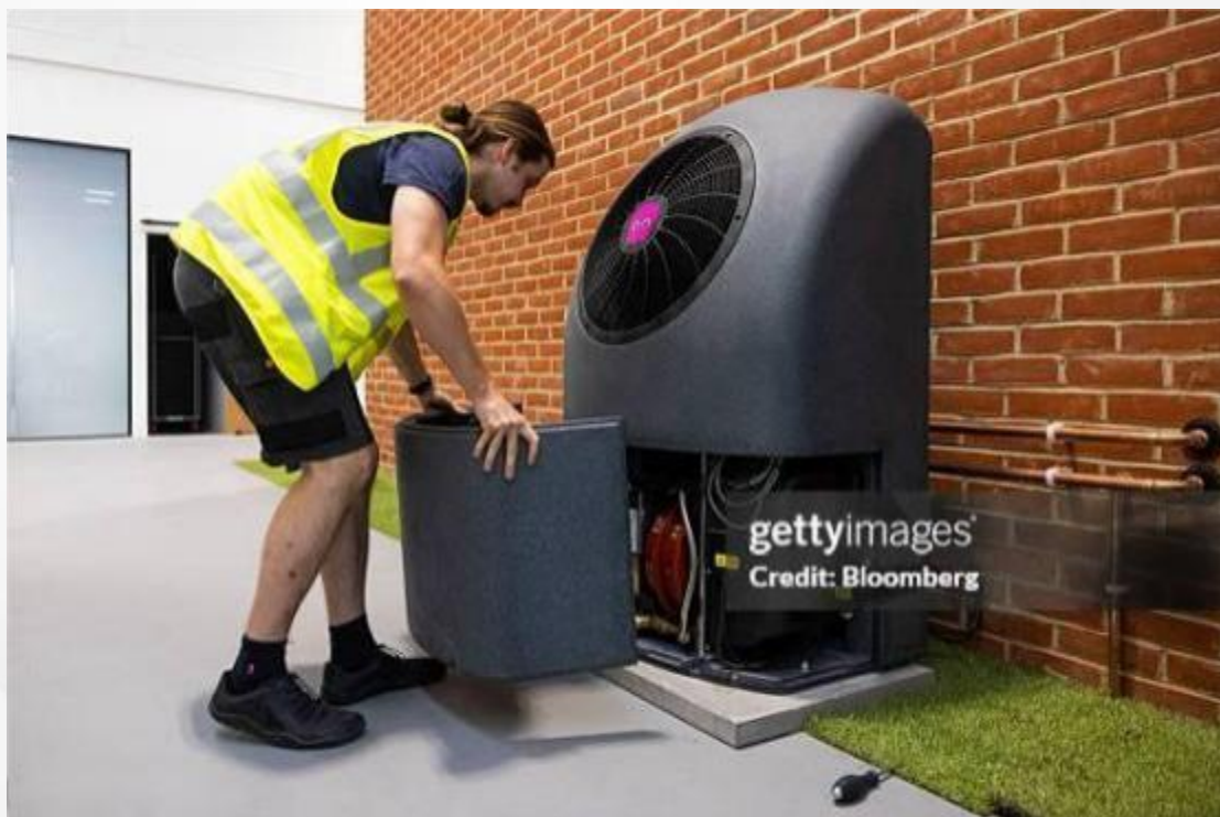
Actual application scenarios of heat pump installation
